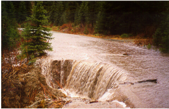
Road failures are a common problem on FS lands, especially after storm events. Flathead NF photo
